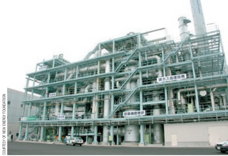
The carbonized sewerage sludge facility of the Bureau of Sewerage, Tokyo Metropolitan Government, praised for the efficiency of its energy systems and for converting sludge into a resource.
