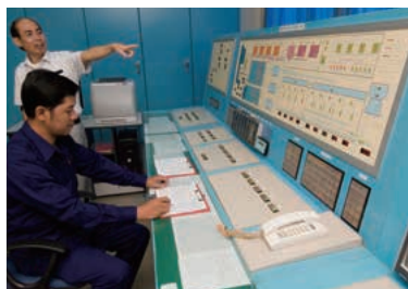
The monitoring room at the Phum Prek Water Treatment Plant in Phnom Penh, where the system is monitored around the clock.
