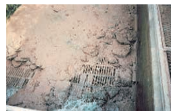
Photo from around 1993 of the neglected filtration pond at water treatment plant.
