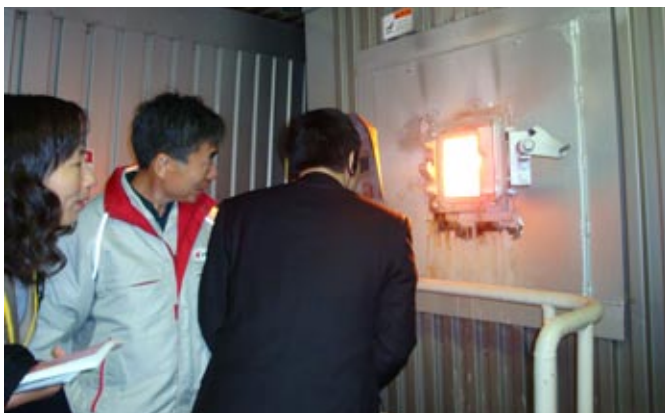
Visitors from China look inside a boiler at the Electric Power Development Co.'s Isogo Thermal Power Station in Yokohama, Kanagawa Prefecture, as part of ongoing Japan-China co-benefit cooperation. This coal-burning station is equipped with some of the world's leading technologies to combat atmospheric pollution.
