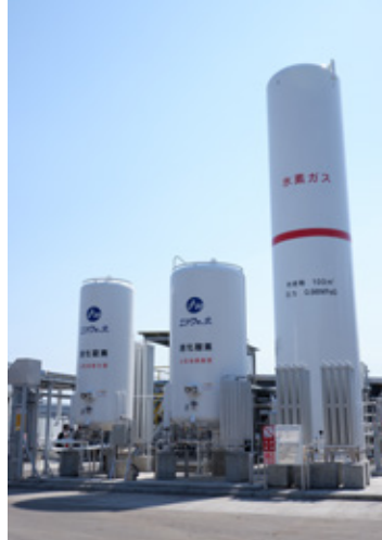
Hydrogen gas holders Photo: Osamu Sawaji
