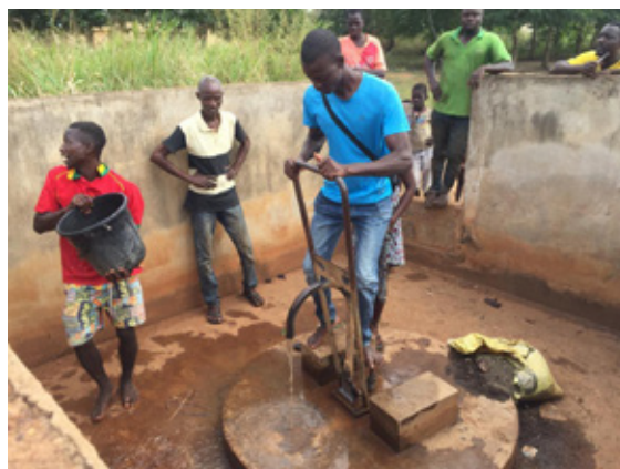
The well repaired through Hyuga-Togo cooperation Photo: Courtesy of the Japan-Togo Friendship Association
