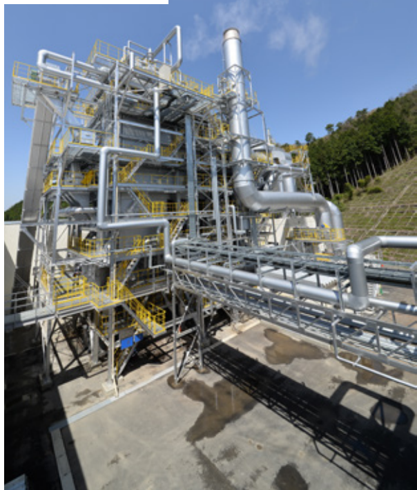
Maniwa Biomass Plant
