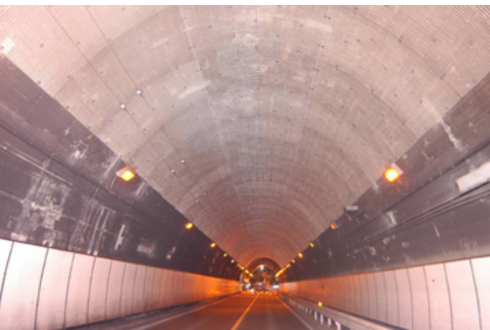
Tunnel walls covered with mesh ARG Fiber Photo: Courtesy of Nippon Electric Glass Co.,Ltd.
