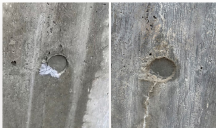
A self-healed (right) crack in a block of concrete
